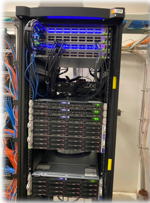
A rack of 2x2 SDN fabric, CPU (and GPU) servers at each edge location forming the edge cloud
